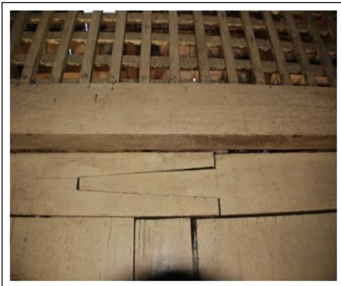
Figure 8: Wall joint of Kampung Tuan Mosque.
