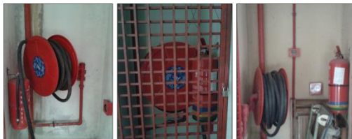
Figure 15: No provision of fire safety sign for each fire extinguisher
