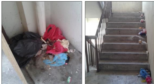
Figure 16: Garbage scattered around lift lobby and staircase
