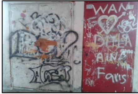
Figure 14: Fire indication sign covered by graffiti
