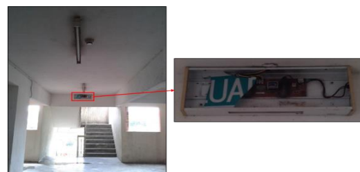
Figure 13: Vandalized emergency exit sign
