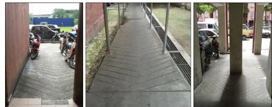
Figure 17: Ramps without handrails
