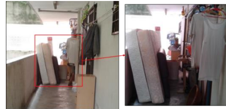
Figure 12: Escape route blocked by mattresses and other items
