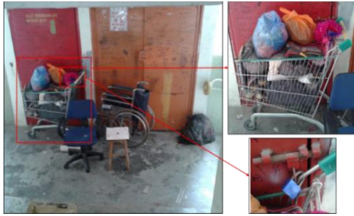
Figure 10: Trolley, chair and wheelchair blocking access to fire-fighting equipment
